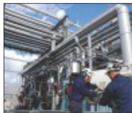
Industrial Water Supply
